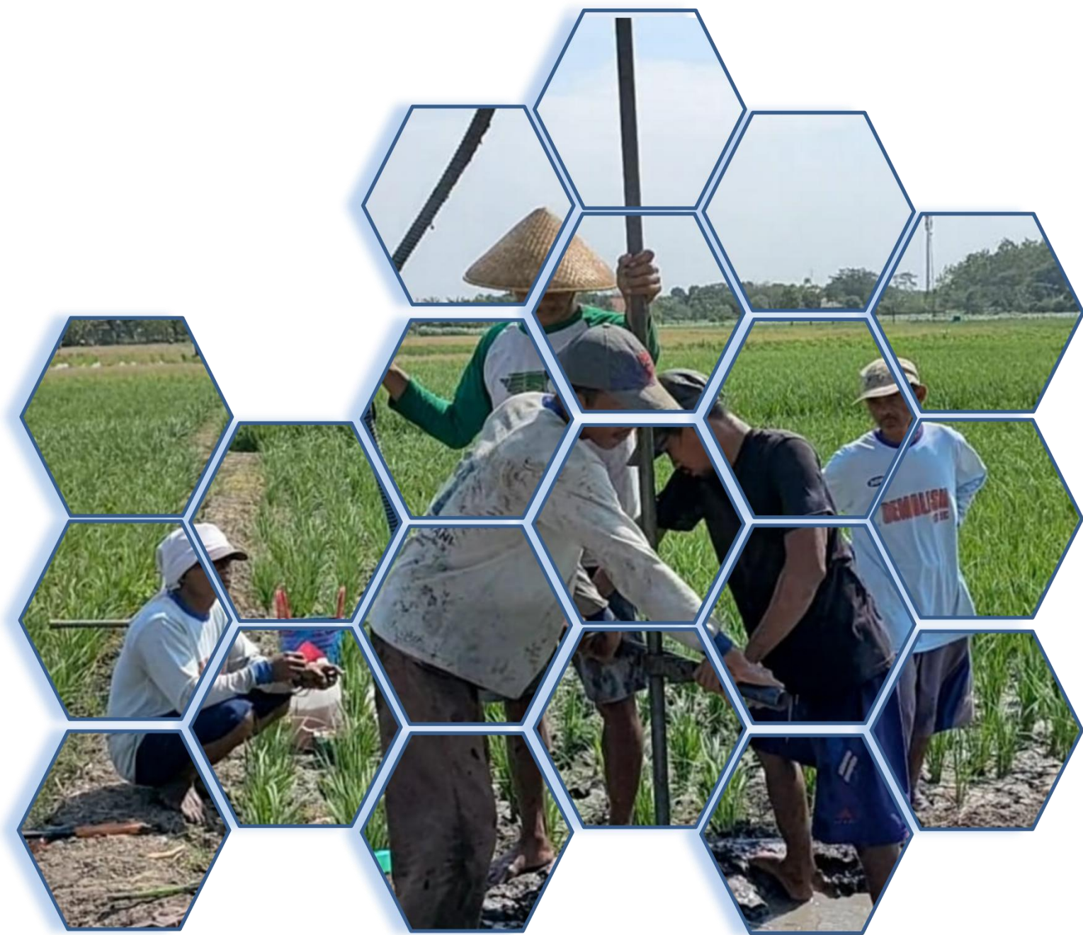
Water well crew drilling & installing a water well for Rice Field Farmers.
